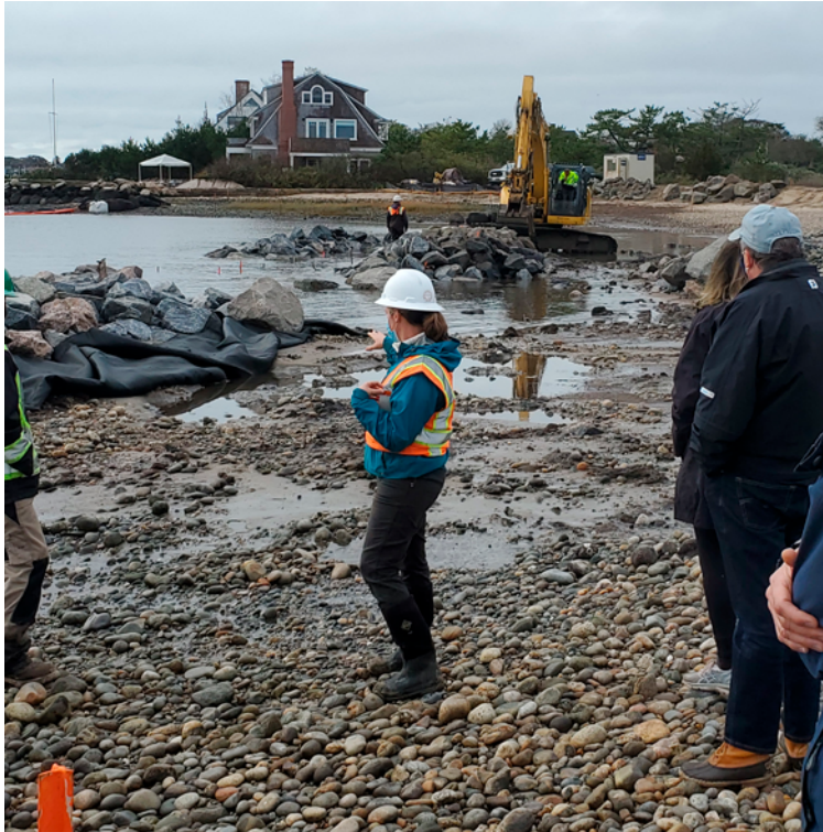
FIGURE 5.10 Construction of rock sill along Fenwick Point in Old Saybrook. Photo: Juliana Barrett
