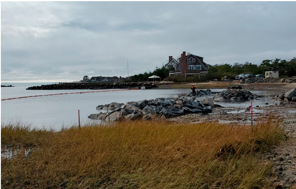
FIGURE 5.11 Completed rock sill along coastline of Fenwick Point in Old Saybrook. Photo: Juliana Barrett
